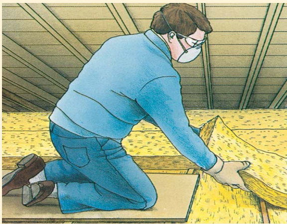
INSULATING WITH UNFACED BLANKETS: Begin laying the blankets at the outer edges of the attic and work toward the middle.
